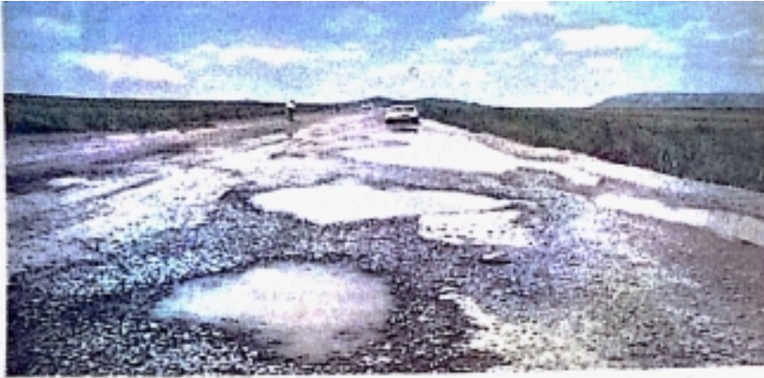
In the Free State near Sterkfontein Dam, there is some road in the potholes.
